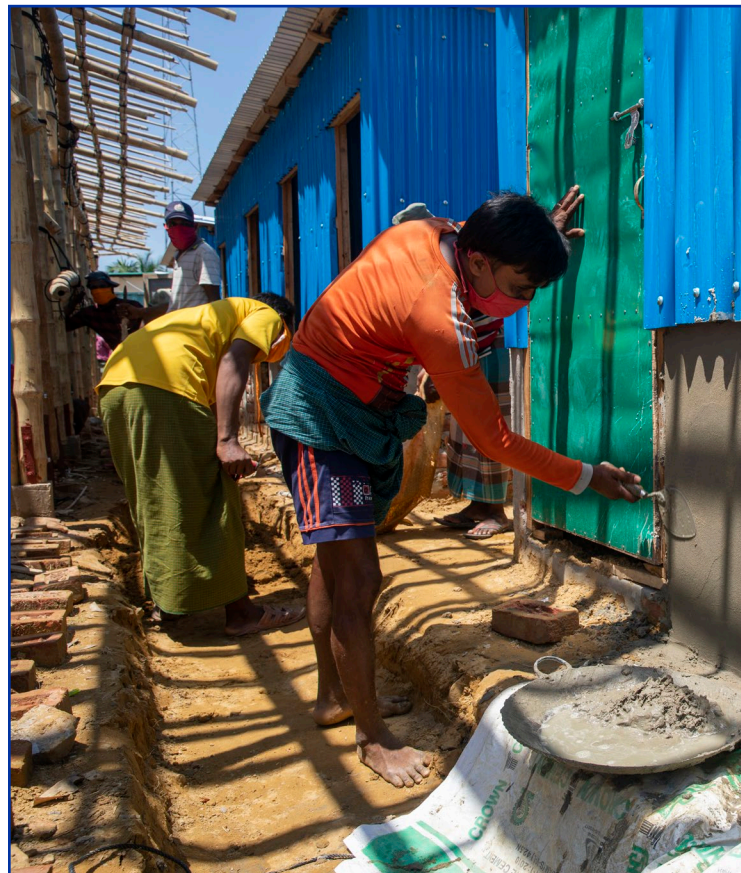
Community members are employed by IOM to construct and renovate isolation and treatment facilities in Cox's Bazar, Bangladesh.
