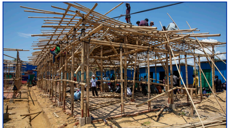
Community members are employed by IOM to construct and renovate isolation and treatment facilities in Cox's Bazar, Bangladesh.
