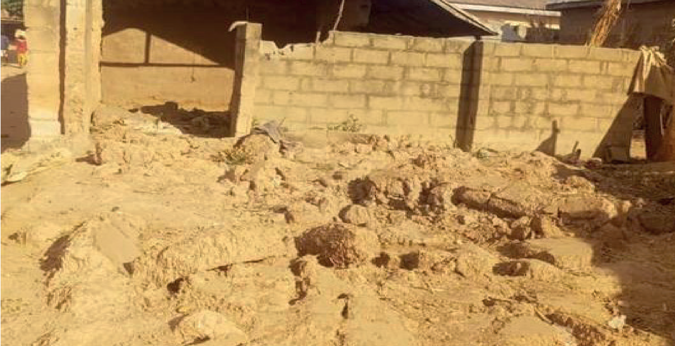
A shelter in ruins after the flooding in Funakaye LGA of Gombe State © IOM Nigeria / Alimi JOEL
