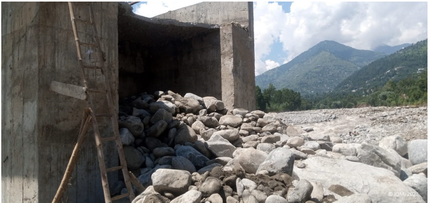
Figure 4: Damaged house in Chitral, Khyber Pakhtunkhwa.
