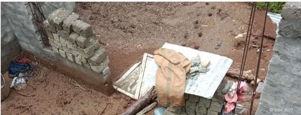
Figure 3: House damaged in village Danin Gol, Lower Chitral, Khyber Pakhtunkhwa.
