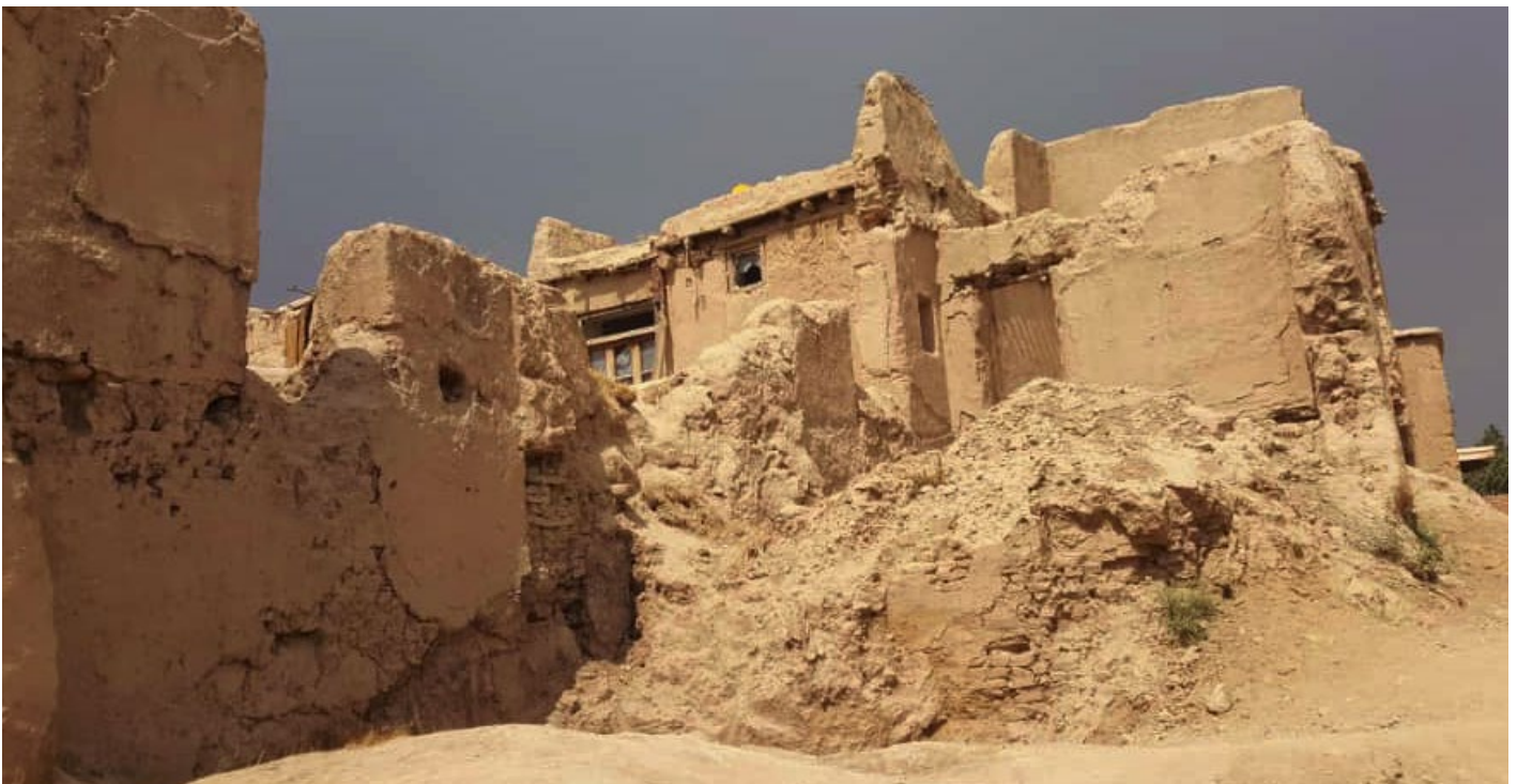
20% of all houses in Kabul are either severely damaged or completely destroyed. Both conflicts and natural disasters have severely affected livelihood opportunities and housing in Kabul. © IOM 2020
