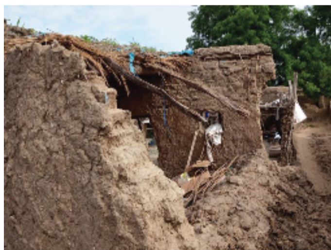
A Damaged House in Gujba, Gujba LGA
