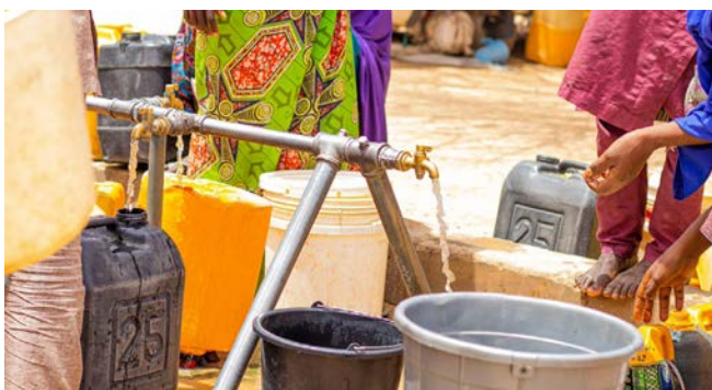
Potable water in Gubio camp, Gubio ward of Maiduguri Metropolitan Council, Borno State © IOM Nigeria/A. Phoebe/ IOM 2021
