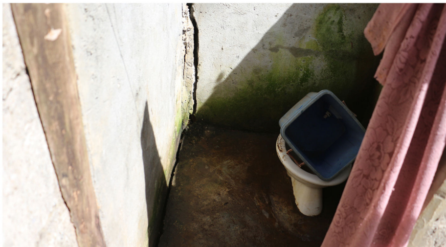
Balo-i: Insufficient useable well lit WASH facilities/ latrines with doors.
