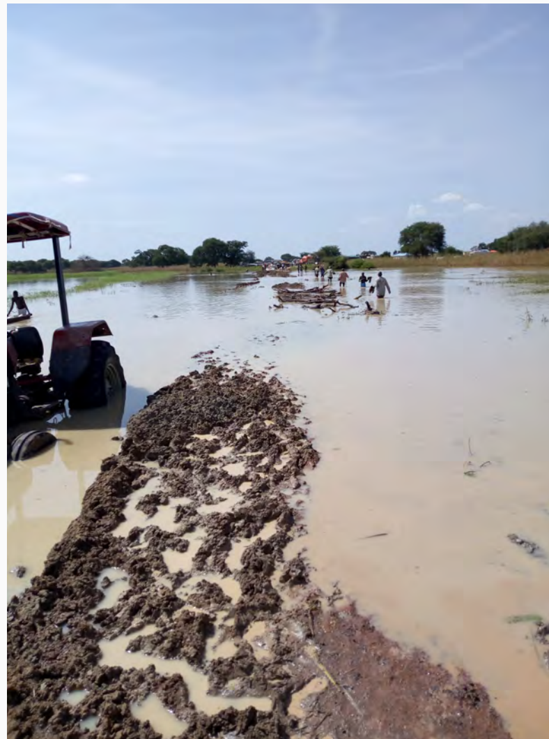
Banton Bridge, where roads from Unity, Northern Bahr el Ghazal and Western Bahr el Ghazal meet, passing through Agok (Abyei Admin. Area) in direction of Abyei Town to Amiet Market. The road is frequently flooded limiting traffic between Sudan and South Sudan. 28 September 2018, © IOM, DTM
