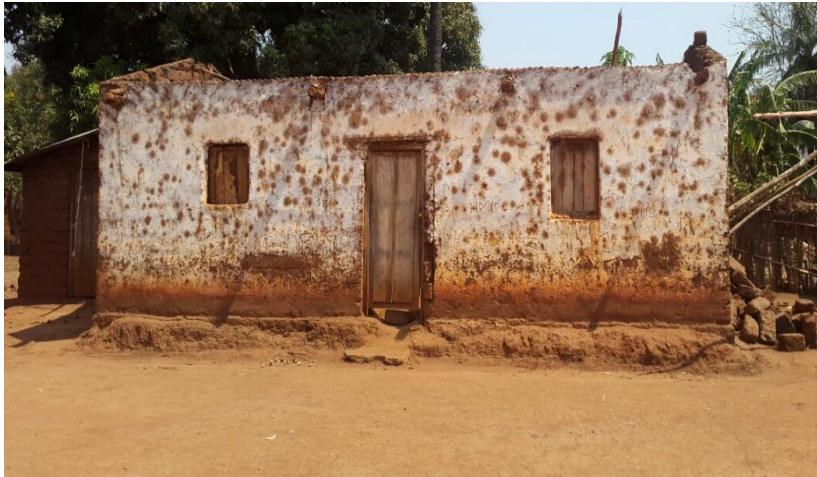
Picture 4: Rain damaged house – Ruyigi province– September 2016 – Credit: IOM Burundi
