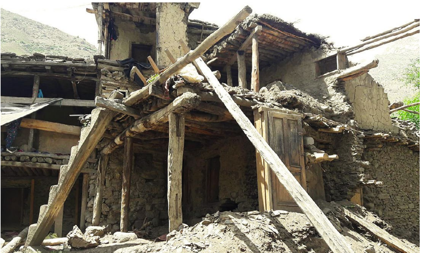
Return IDPs often return to find their homes and possessions damaged, destroyed or stolen — such as this house in Nuristan — which was destroyed during clashes between government forces and anti-government elements. Destroyed homes pose an immense challenge to reintegration, as income levels drop and significant debt is accrued during displacement, limiting IDP's opportunities to find alternative housing. © IOM 2018
