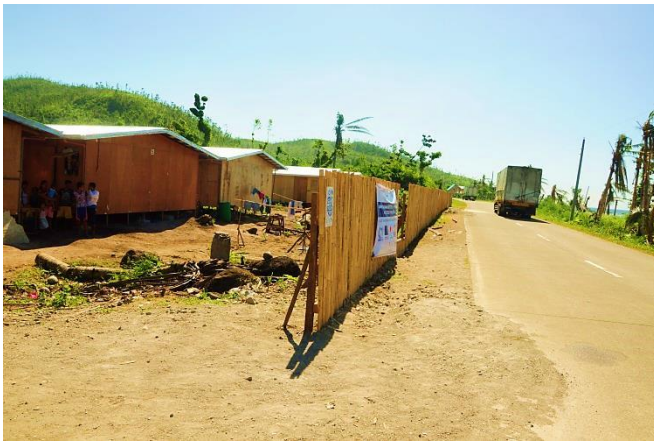
Fencing of the site perimeter near roads prevents accidents from happening especially children. Marabut Bunkhouse, Western Samar
