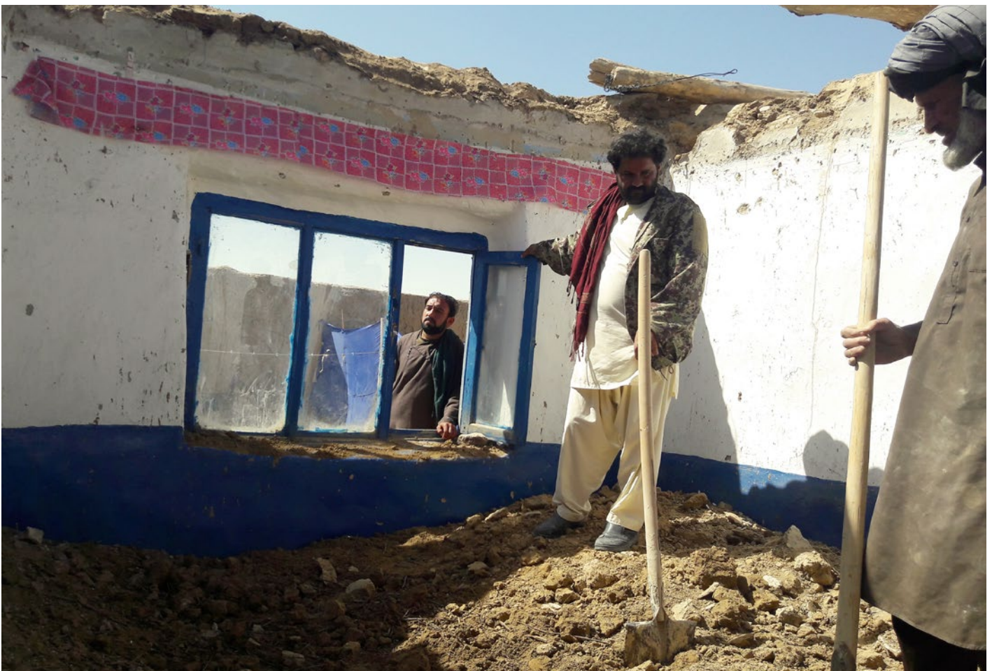
Both conflict and natural disaster have severely damaged houses in Ghazni, many houses are moderately — and some are completely — destroyed. This returnees' house was heavily damaged during heavy rains in Muqur district. © IOM 2018
