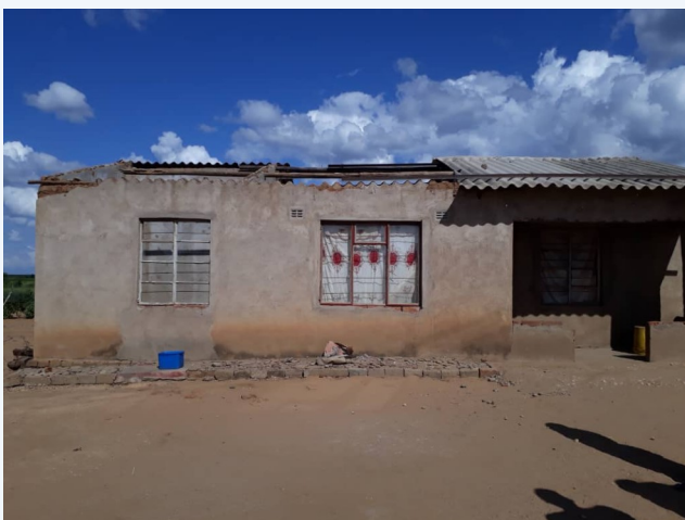
Damaged house in Chiredzi Rural District ward 6
