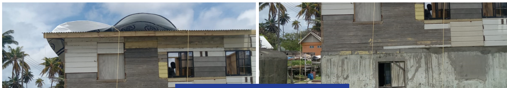
HOUSE DAMAGE IN BEQUIA © TARAJI FOUNDATION 2024
