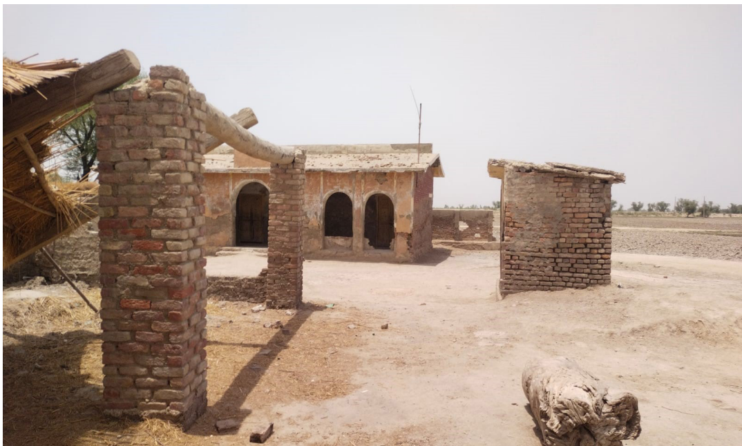
Damaged shelter in Sindh © IOM 2023
