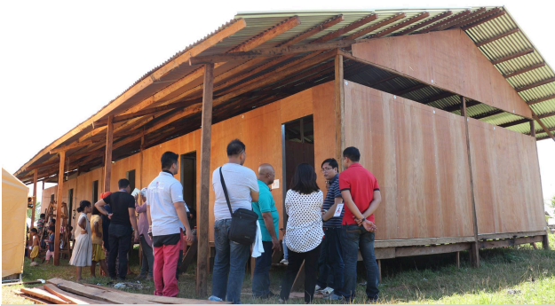
USec. Yano of Task Force Bangon Marawi visits the Alternative Dwelling Spaces (ADS) being constructed by IOM at the Madrasah Markazi, Balo-i, Lanao del Norte, to provide alternative shelters to IDPs currently living in tents.
