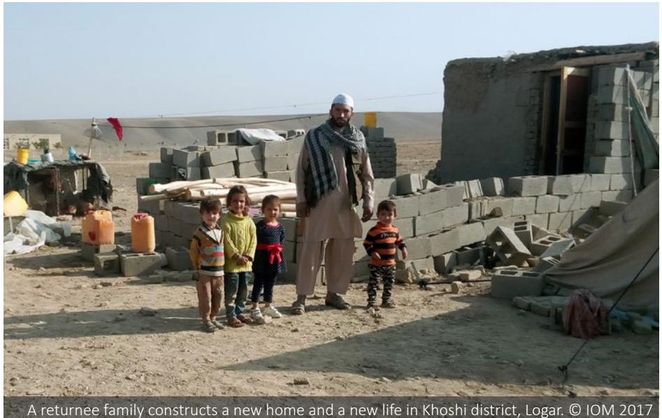
A returnee family constructs a new home and a new life in Khoshi district, Logar. © IOM 2017
