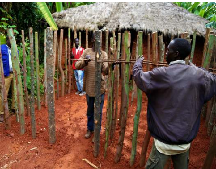
Photo 4: Construction of a temporary shelter for an IDP whose house was completely destroyed by torrential rains. Ngozi province, Kiremba commune © IOM 2018.
