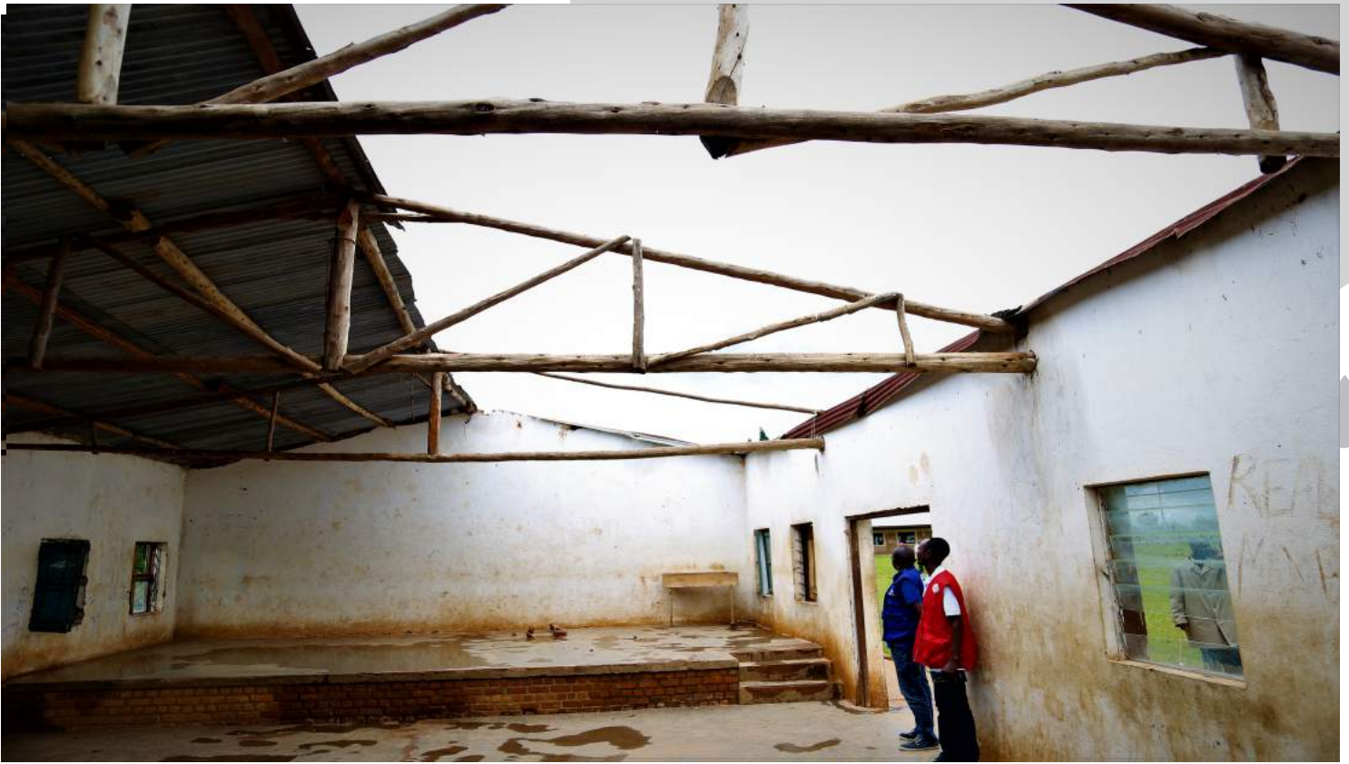
Photo 3: Large hall damaged by torrential rains and strong winds. Bururi province, Rutovu commune © IOM 2018.
