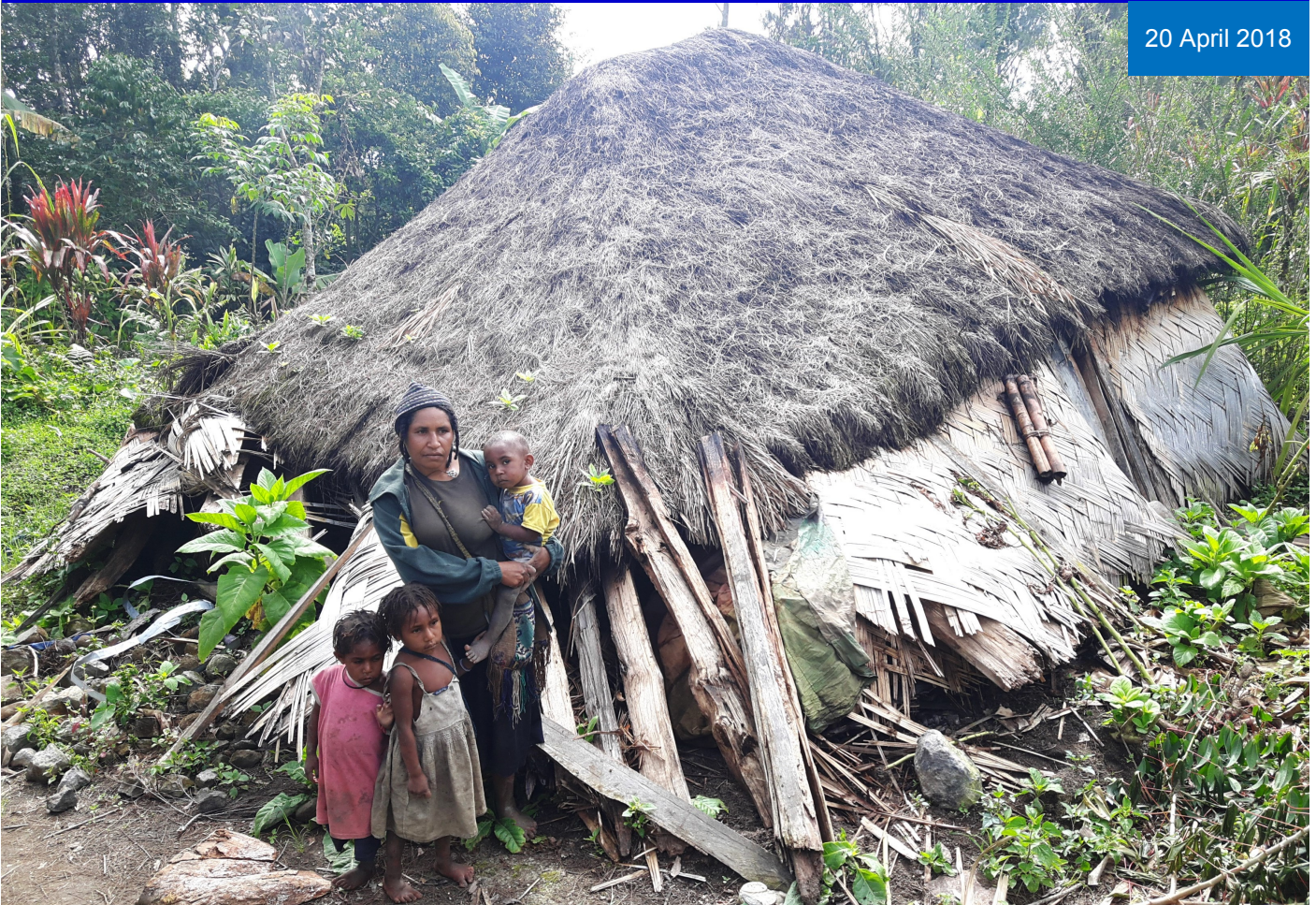
An IDP family at their house damaged by the earthquake in Puren, Hela © Peter Murorera. IOM/ UN Migration Agency
