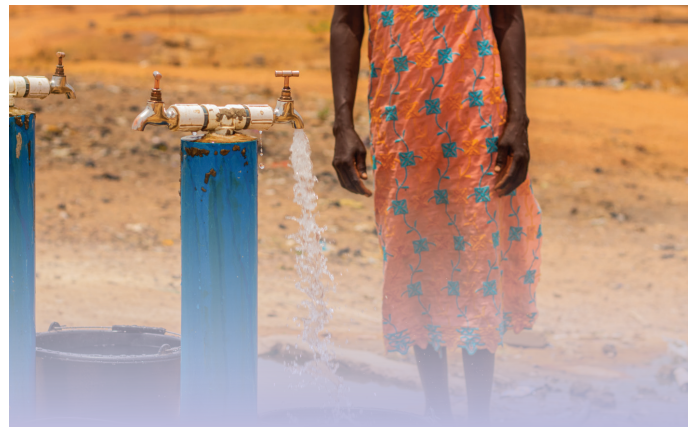
To improve the well-being of IDPs in North-east Nigeria, IOM continues to provide coordinated humanitarian response by setting up WASH facilities in camps and camp-like settings. Borno State © IOM Nigeria 2022
