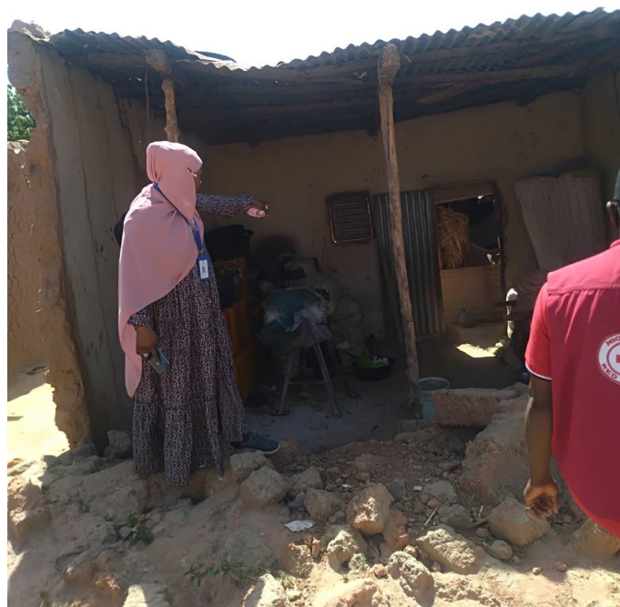
A building affected by heavy rainfall in Katsina State. © IOM 2021 / Mohammed ALIYU.
