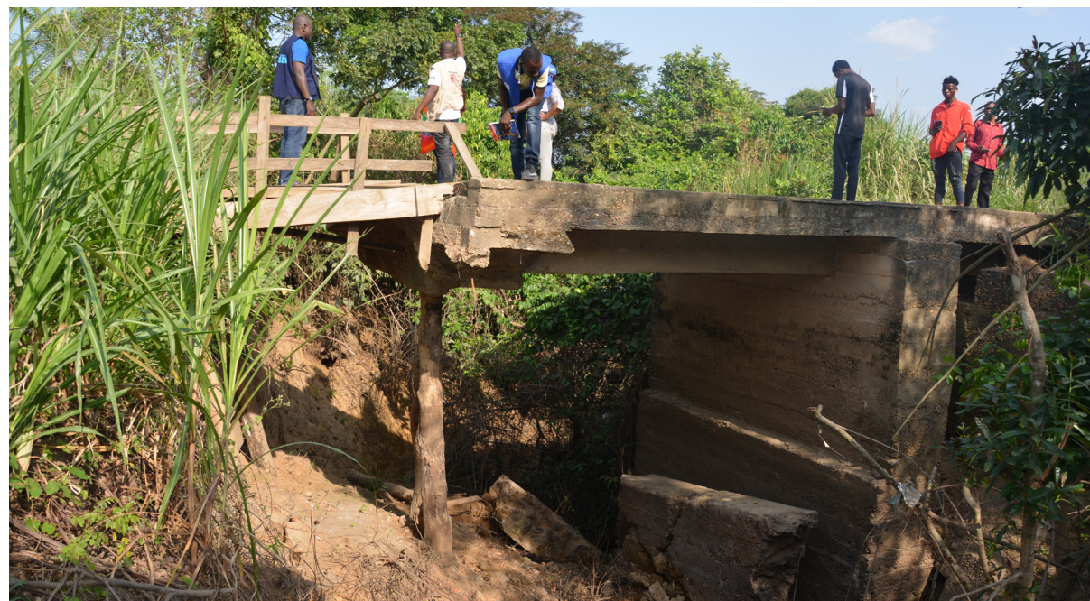
Damaged bridge as a result of flooding in Ahaha community, Ovonum ward, Obubra LGA of Cross River State © IOM Nigeria/MIDIGA Lagu/ IOM - November 2022
