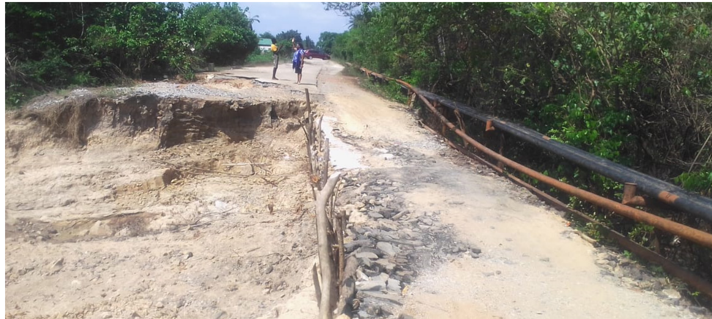
Flood damage on road leading to Evel Abalangada, Ward 5, Ndukwa East LGA © IOM Nigeria/Miriam/IOM 2022
