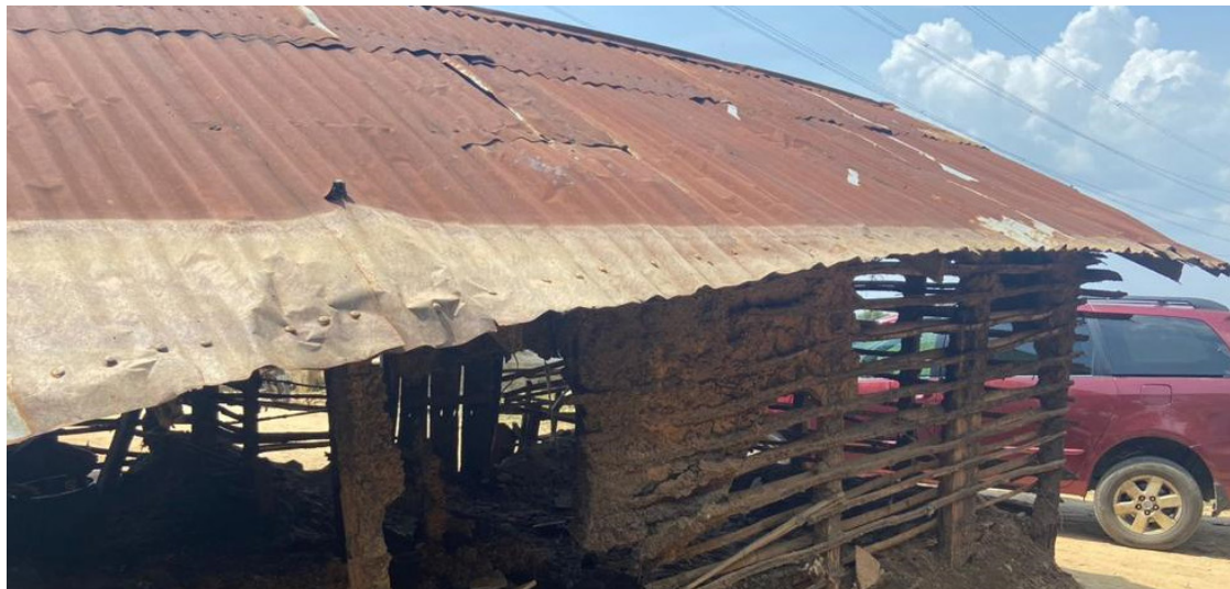
Flood affected shelter at Oko Power Line site © IOM Nigeria/Michael/IOM 2022
