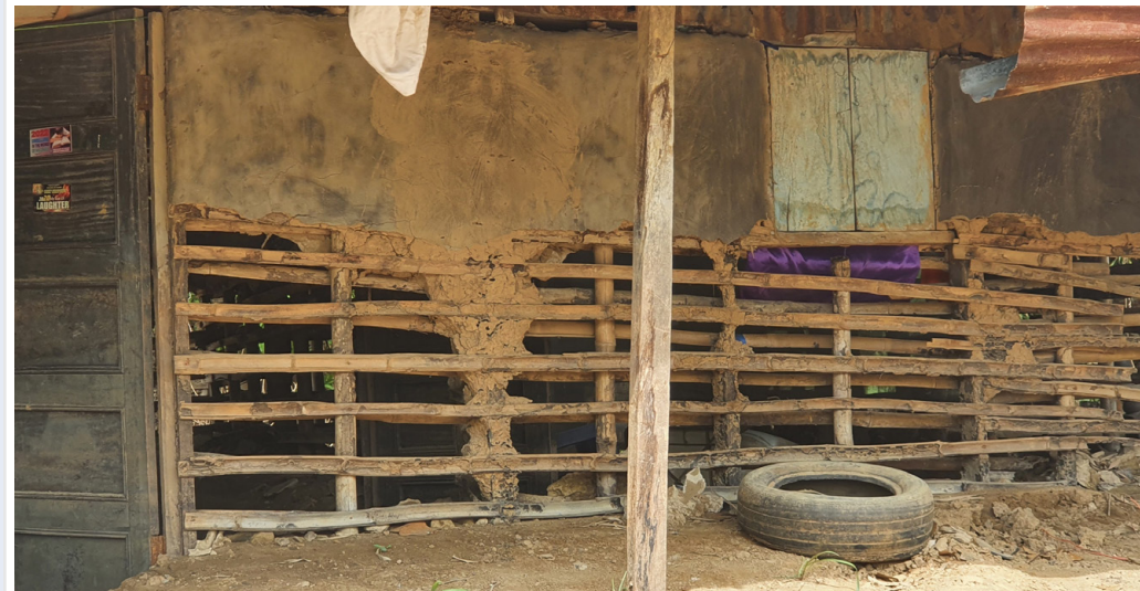
Post flood effect on communal structures in Elenchele site, Ward 11, Oshimili LGA © IOM Nigeria/Miriam/IOM 2022
