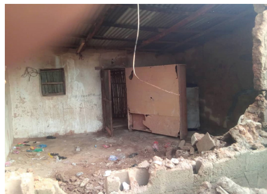
Damaged structure in Yan Kanwa Ramin Kasa ward Potiskum LGA.
