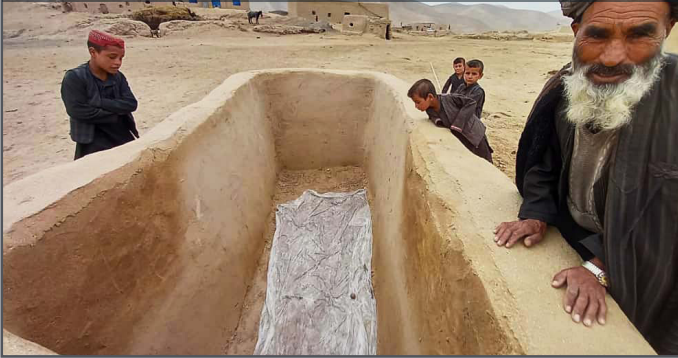
A community in Jawzjan province constructs a storage vessel to collect rainwater during the winter. Water needs are high in Jawzjan province, where 108,294 IDPs and returnees from abroad do not have access to safe drinking water. © IOM 2021
