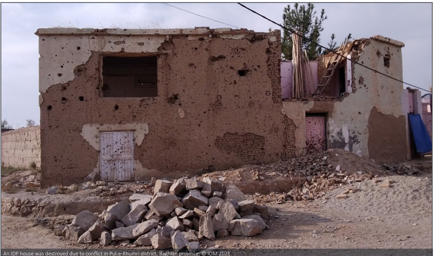
An IDP house was destroyed due to conflict in Pul-e-Khumri district, Baghlan province. © IOM 2021
