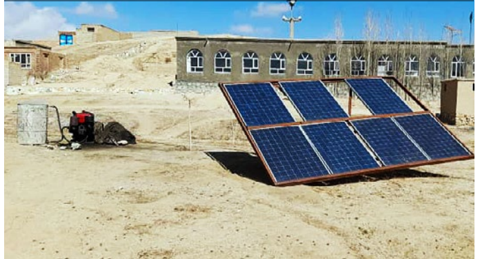
This community in Ghazni province has installed a solar-powered water pump to sustain their water needs. © IOM 2021
