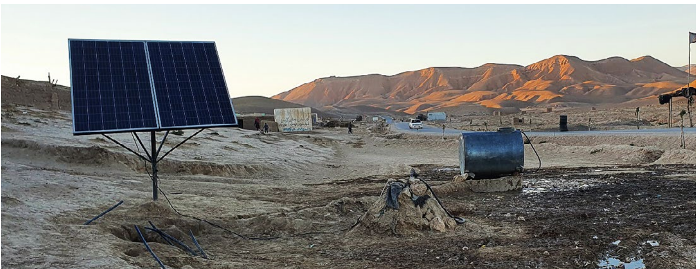
This community in Sar-e-Pul province has installed a solar powered water pump to sustain their water needs. © IOM 2020
