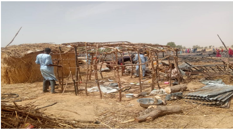
Residents of Gongolong Kareram Camp re-constructing damaged shelter after the fire outbreak©IOM-DTM/2021
