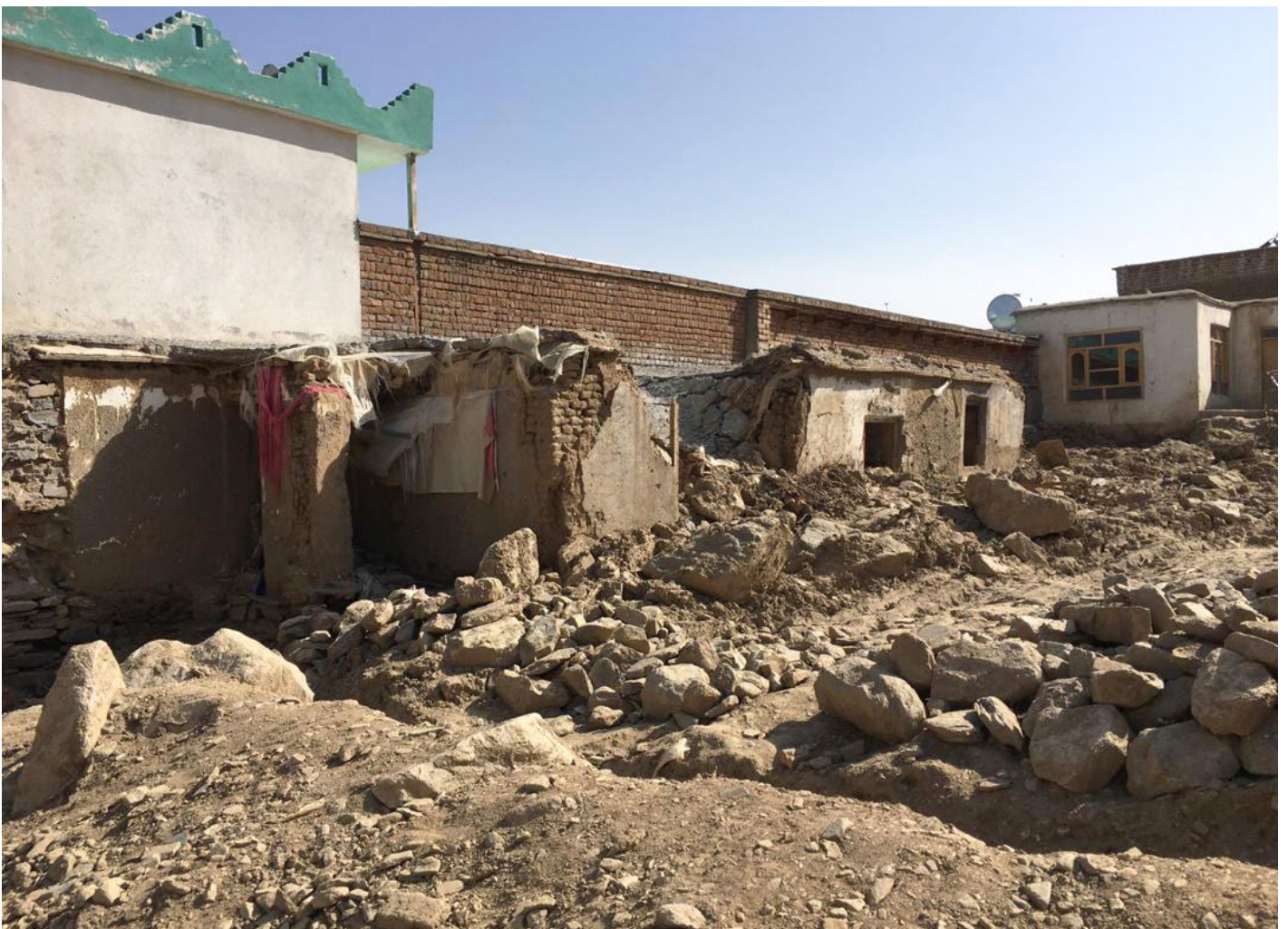
As a result of conflict and natural disaster, 61% of all housing in Parwan is either damaged or destroyed, as here in Bagram district. © IOM 2020
