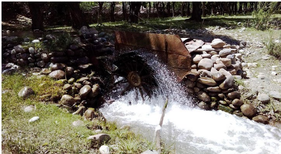
This community in Panjsher has installed a turbine to generate power and supply electricity to local communities. © IOM 2020
