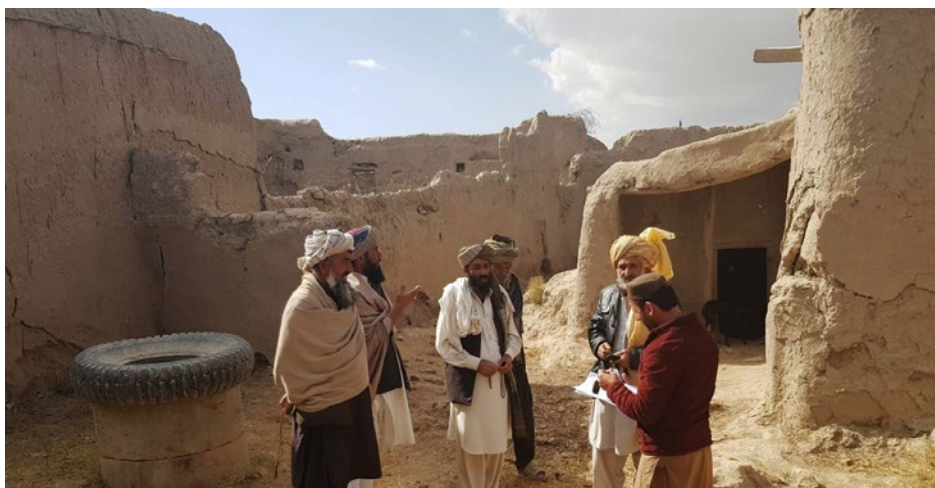
Shelter needs are high in Paktika, where 523 IDPs and returnees live in tents or open air. Like these families living in destroyed houses, many houses in Paktika are damaged by both conflict and natural disasters. © IOM 2020
