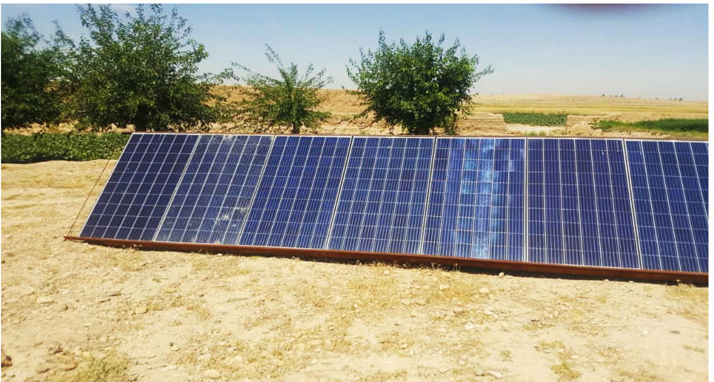
This community in Helmand installed a solar-powered pump to supply water for irrigation. © IOM 2020
